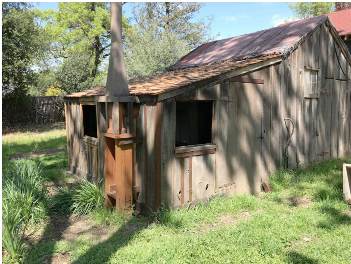
Fig. 2 Wash House (Left Side of Structure) in mid-restoration 2019. The project was paid for through a Questers Grant with work done by our amazing volunteers from the Presbyterian Church.
